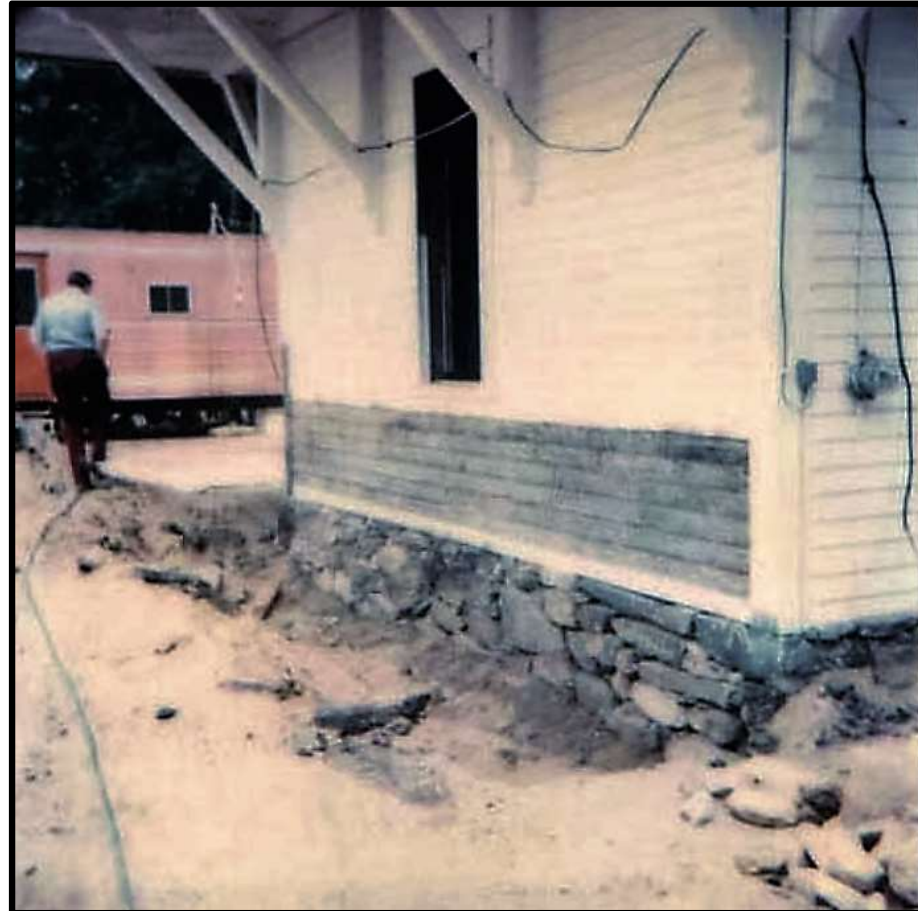
Image Number 13 West end elevation circa 1977 showing original rubble stone foundation masonry.
